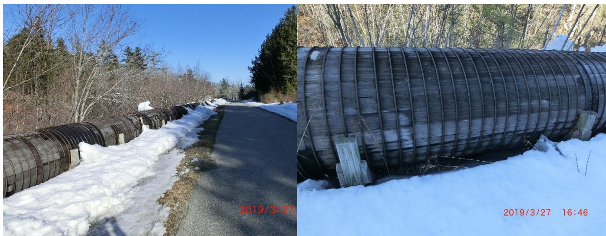
Photo 2-6 Wood Stave Penstock
