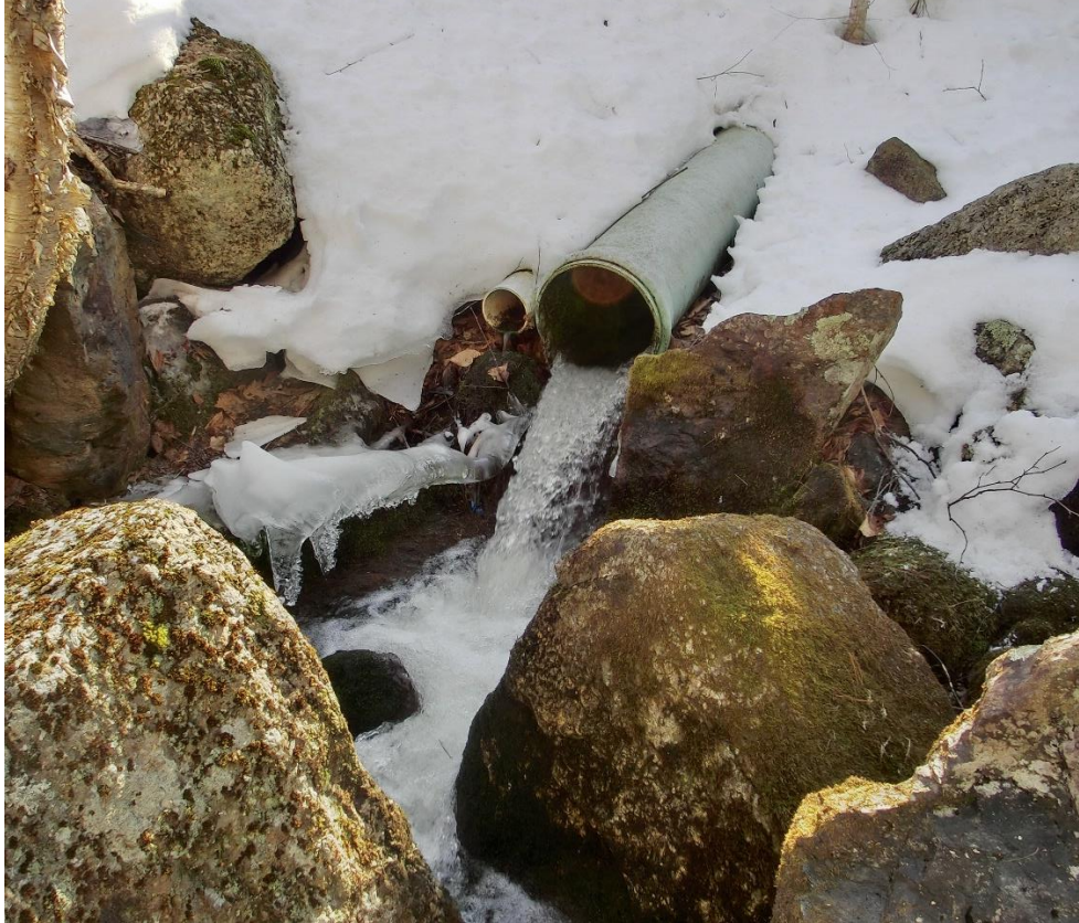
PHOTO 3-6 GLNFH FILTER OVERFLOW DISCHARGE INTO REEDS BROOK
