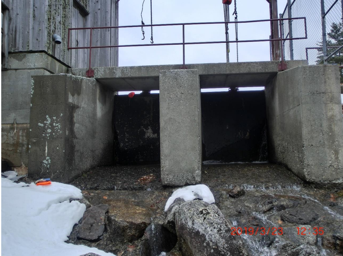
PHOTO 4-5 GREEN LAKE DAM GATES
