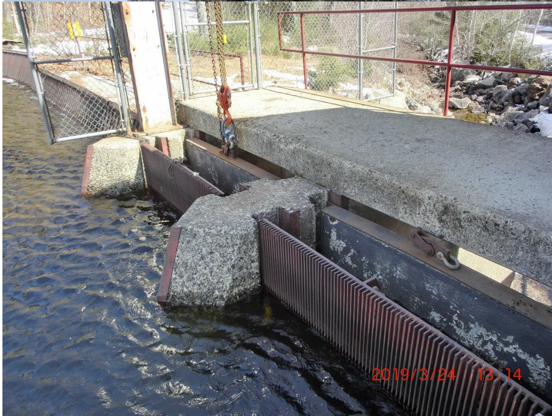
Photo 2-4 Green Lake Dam Gates
